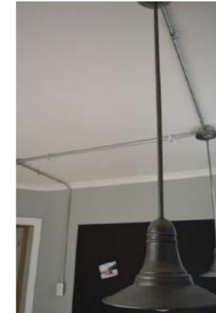
Surface mounted exposed electrical conduit for bench table seating ONLY
